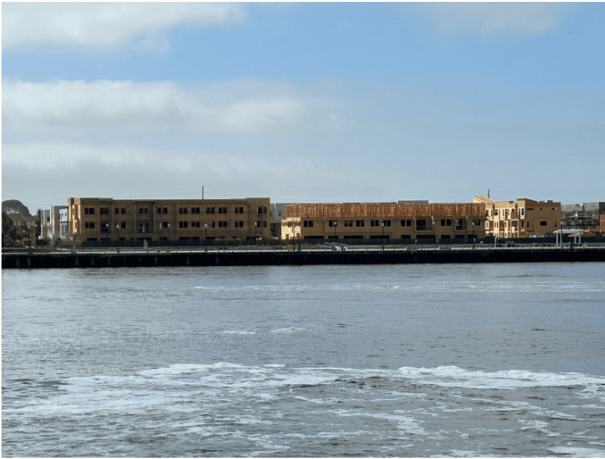
Hundreds of new units of housing under construction in Alameda along the Northern waterfront. Photo Adam Gillitt.
